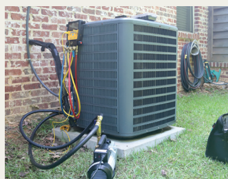
Pre-season HVAC tune ups
